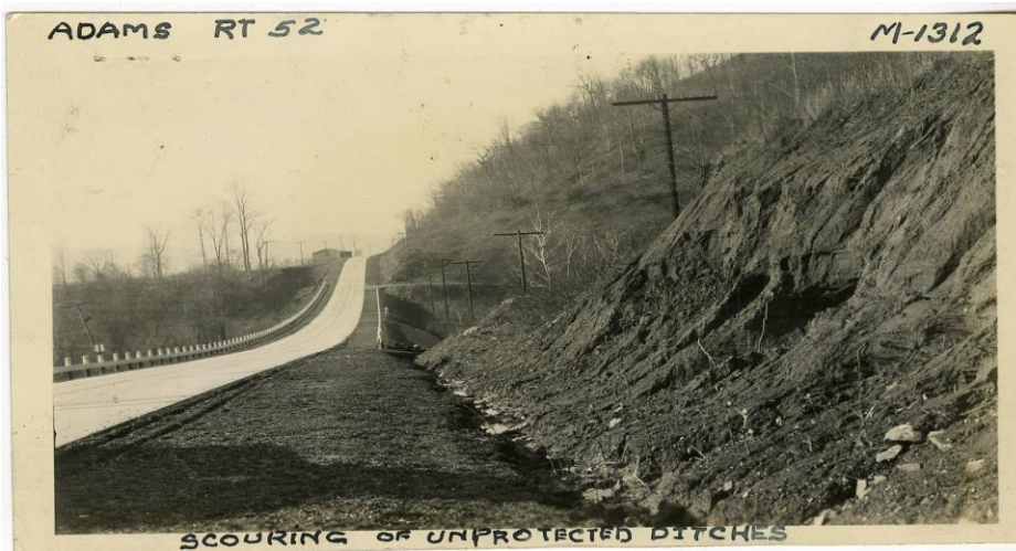
A photo from the Ohio Department of Transportation archives. This photo from 1936 shows scouring of unprotected ditches along SR 52 in Adams County.
